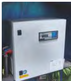
STP Compressor Panel & Water Treatment Plant
